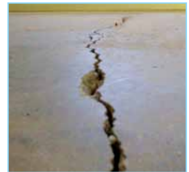
fig. 3) Damage caused by frost heave.
