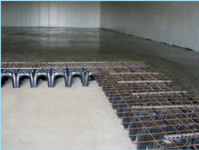
fig. 16) REGGIO EMILIA • Refrigerated Warehouse 6240 m 2
