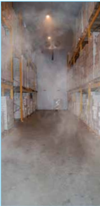
fig. 1) Inside of a freezer room.
